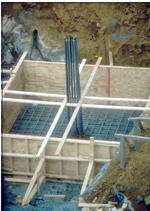
Keep rebar off the grade
