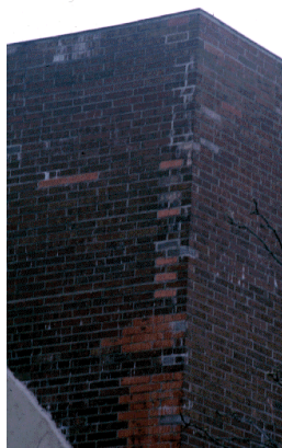
The corners of the cooling tower enclosure were patched with some not-very-close-to-matching brick....
