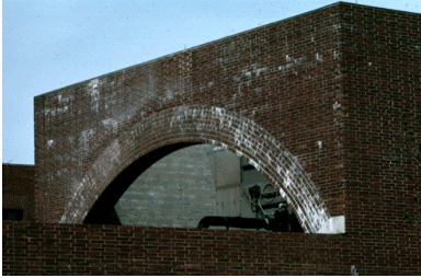
The worst case for the masonry was where it was exposed to moisture from both sides. What does the cooling tower behind this arch produce? How often?
