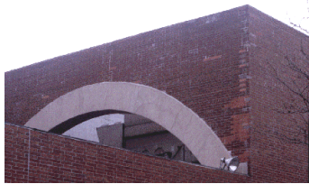
This arch was deemed too badly damaged, and out of sight so it was covered up with cement stucco. How is the stucco doing?
