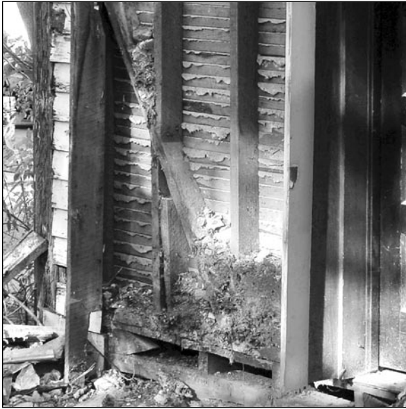
Fig. 14. Down-brace for first-floor wall assembly at 209 Wall Street. Studs cut to fit around brace suggest the brace preceded the wall studs.
