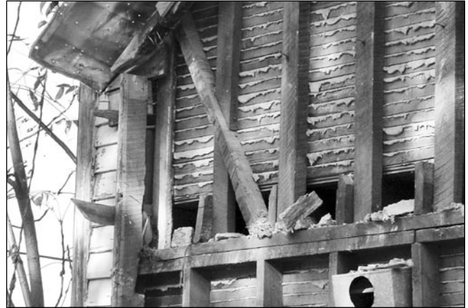
Fig. 16. Down brace for second-floor wall assembly. Studs cut to fit around brace. Joists bear on double top/splice plate.
