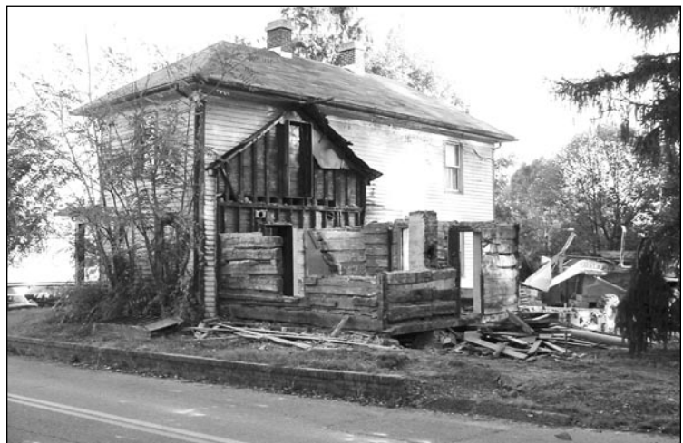
Fig. 12. Log cabin at 209 Wall Street, Blacksburg, VA, in the process of being carefully disassembled for storage and reassembly. I-house with hybrid frame is in the background.
